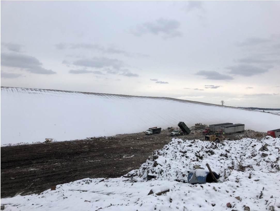
Photo 41: Location 14 – Looking South, Cell 3F Industrial Waste (CCR) Valley Fill Over C&D Disposal Area
